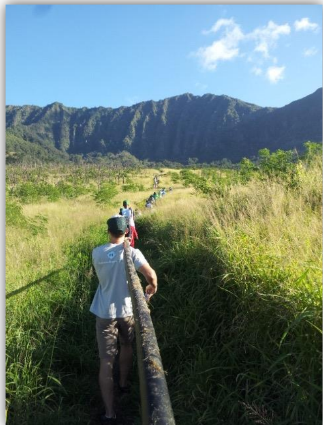
Volunteers carry long sections of pipe to bring water down from a spring.
