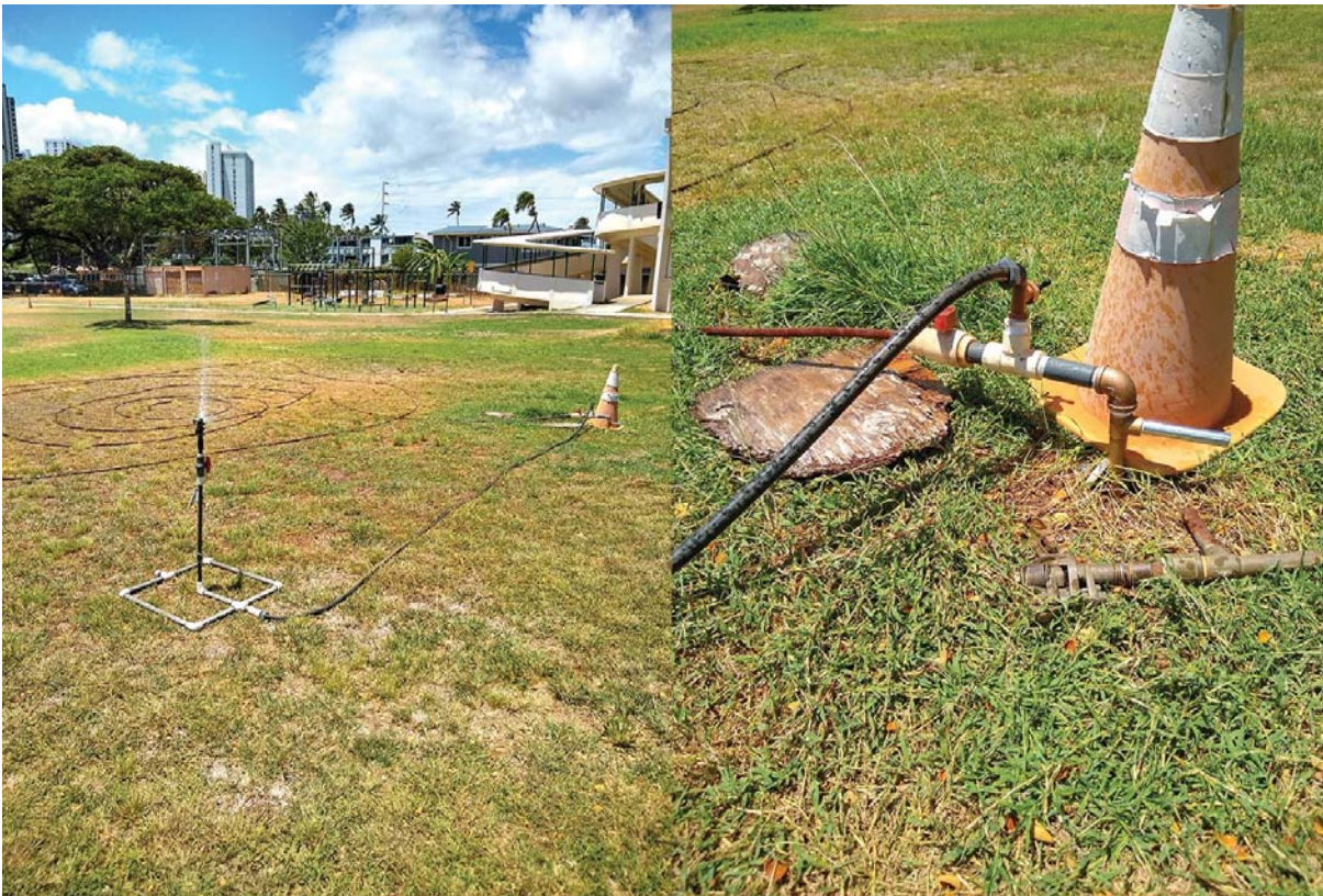
Figure 2. The legacy plug-in irrigation riser system was modified to supply water with both landscape drip tubing as well as overhead sprinkler. Both methods could be used separately or together to provide maximum flexibility with on-campus activities.
