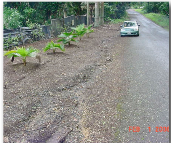
(Before) Roadside ditches are sites of severe erosion, and left untreated can result in road damage.
