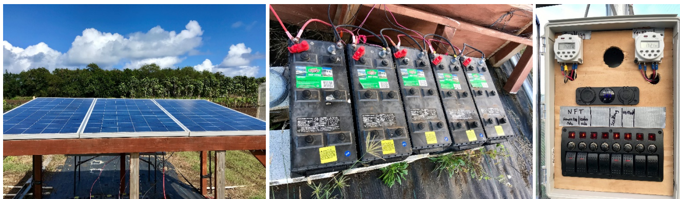
Figure 9. Solar panels, battery bank and electrical panel.
