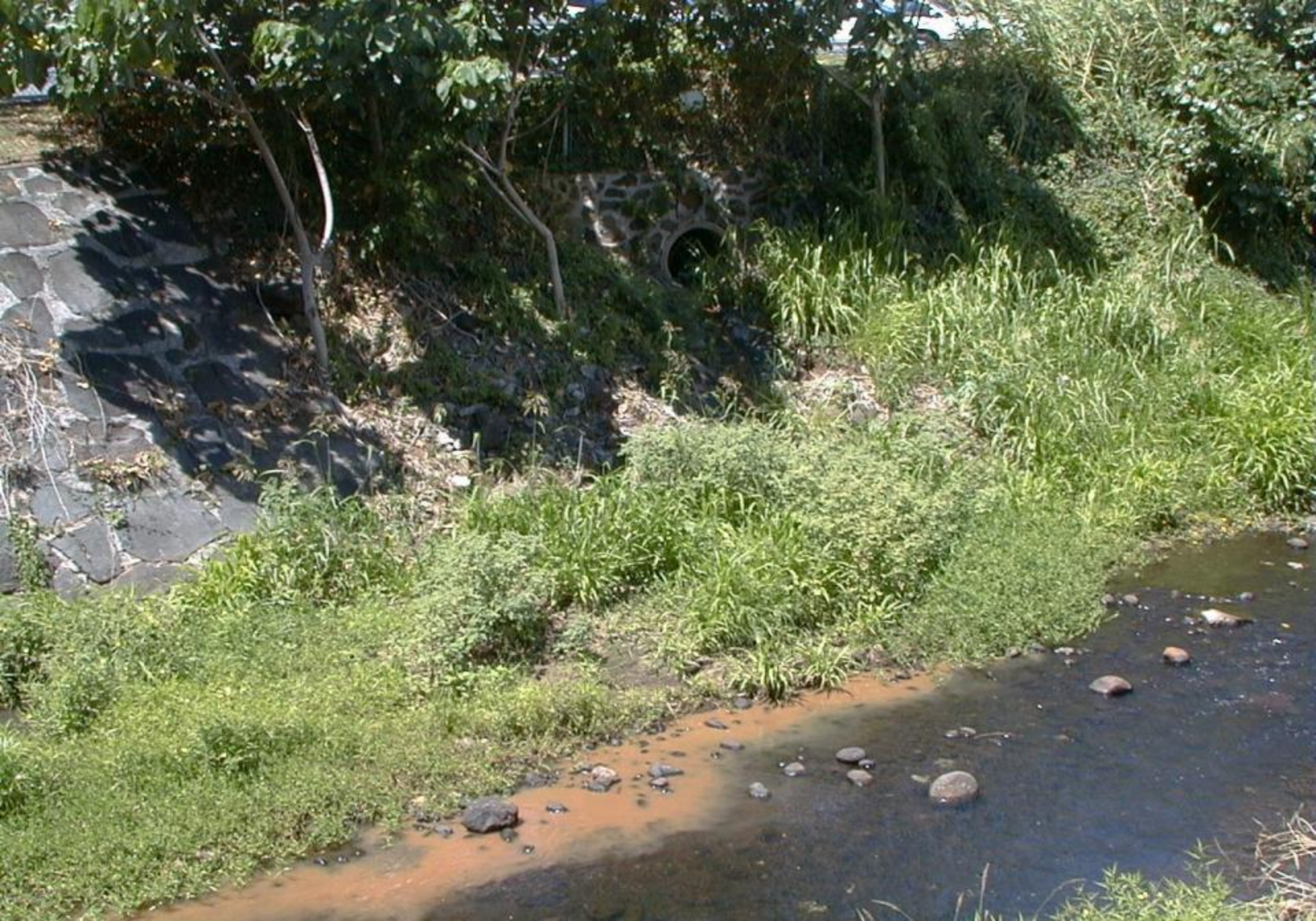
Sediment from culvert – Manoa
