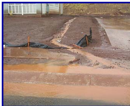
Soil erosion during construction
