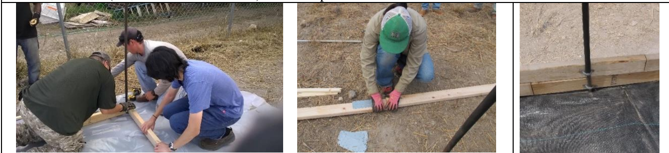
Build the bottom frame with 2"x4" lumber and Simpson's joint plates and secure the bottom frame to each rebar using pipe straps.
