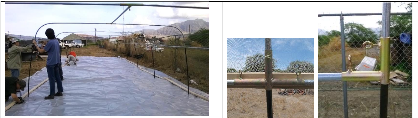
Install rebar at 7'6" spacing, connect bent end of conduit to rebar, join the conduits with the "T" or "L" slide thru EZ Corners ("L" are for the 4 corners). Install top center conduit in front and back of structure.
