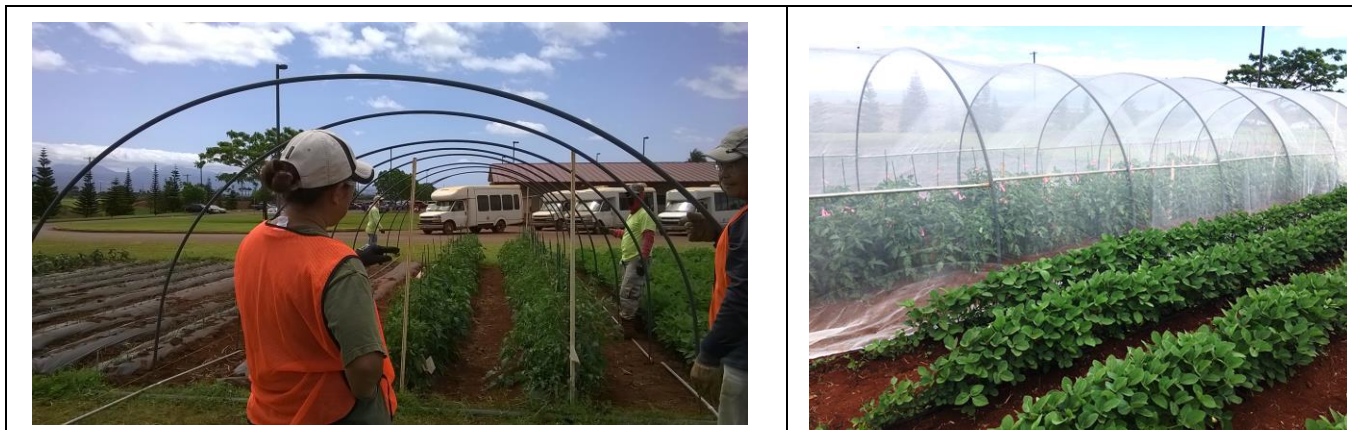
Hoop house structure with rebar and PVC pipes. Spacing conduits on the side provide structural support. Bottom of the screen is then buried with soil.
