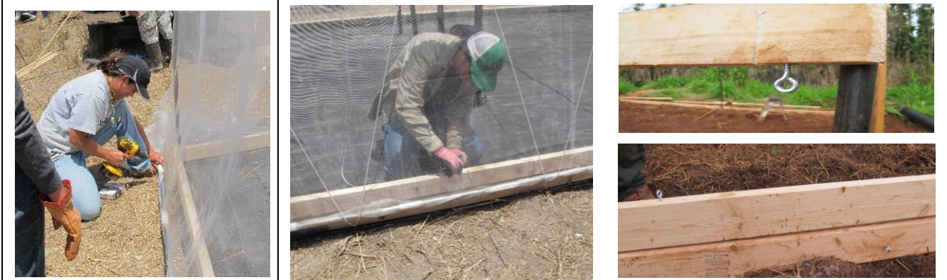
Secure screen of the retracting wall to the conduit, put eye screws on upper and lower wall panel for billow twine.
